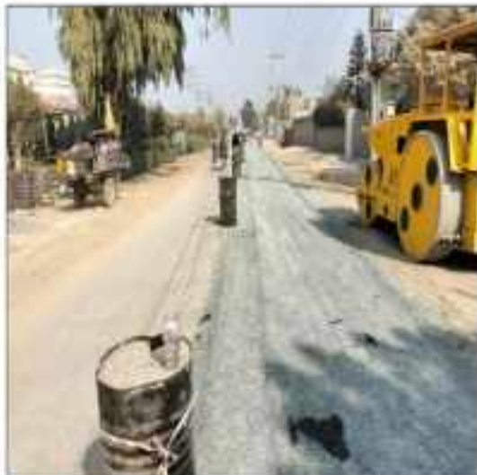
Picture 21: TST is in progress at Kachia Pakka Noor Shah Road under LOT-2
