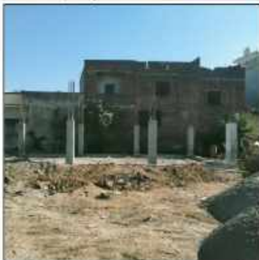
Picture 62: RCC of columns in progress at parking shed Iqbal town Sialkot.
