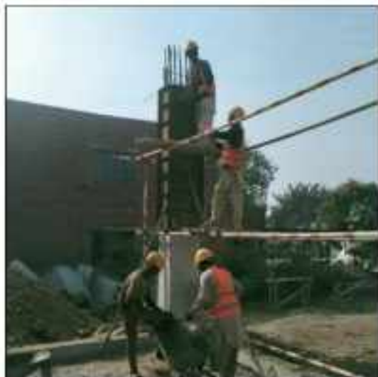
Picture 59: Final pouring of columns in progress at parking shed site Sialkot.
