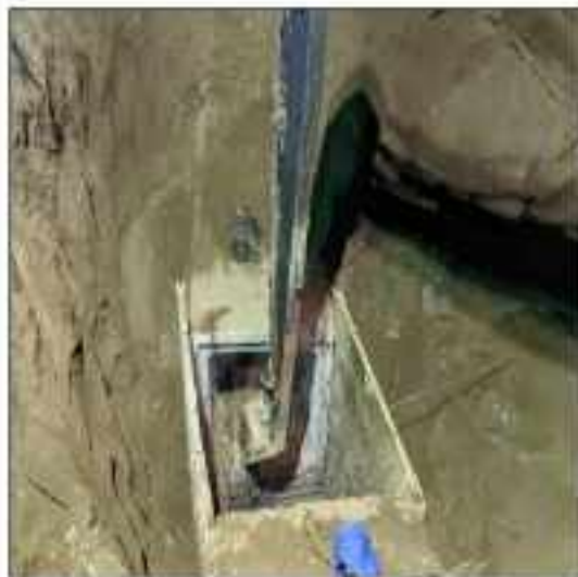
Picture 37: Concrete for BED Slab & Chamber has been started at MH#51 Madina Chowk single cell Conduits line Marala Road LOT-2 Sialkot.
