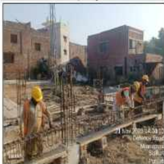
Picture 58: Pile beam construction is in progress at parking shed Iqbal town Sialkot
