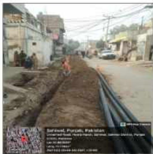
Picture 15: Laying of water supply lines is in progress at LOT-1 Sahiwal
