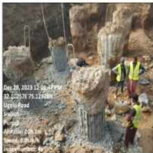
Picture 74: Dismantling of pile up to cut off level is in progress at flyover Sialkot.
