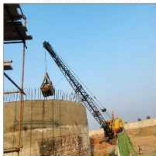
Picture 10: Sinking of collection chamber in progress at Disposal Station LOT-3 Sahiwal.
