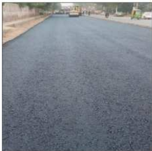
Picture 66: Compaction of Asphalt base course at Iqbal road is in progress.
