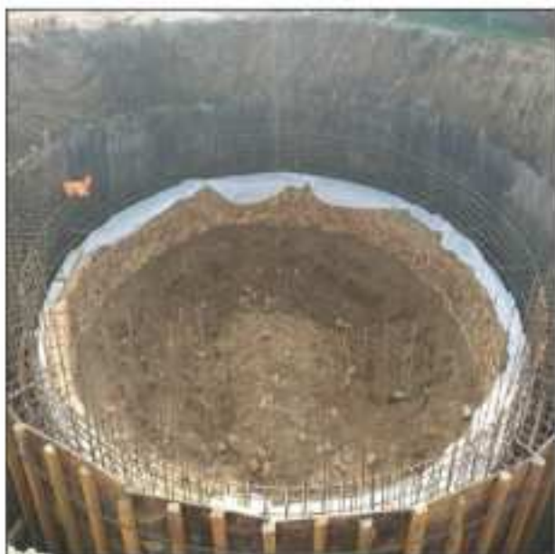
Picture 49: Collection chamber shuttering is in progress at pumping station LOT-3 Sialkot.
