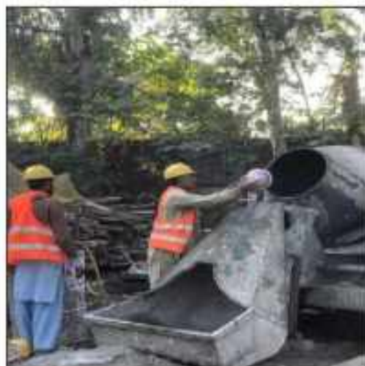
Picture 31: Concrete pouring of overhead water tank T-50 is in progress at Islamic college LOT-4 Sialkot.
