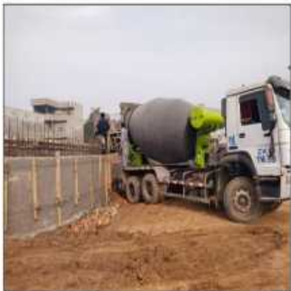
Picture 32: Wet well core wall concrete pouring is in progress at pumping station LOT-3 Sialkot.
