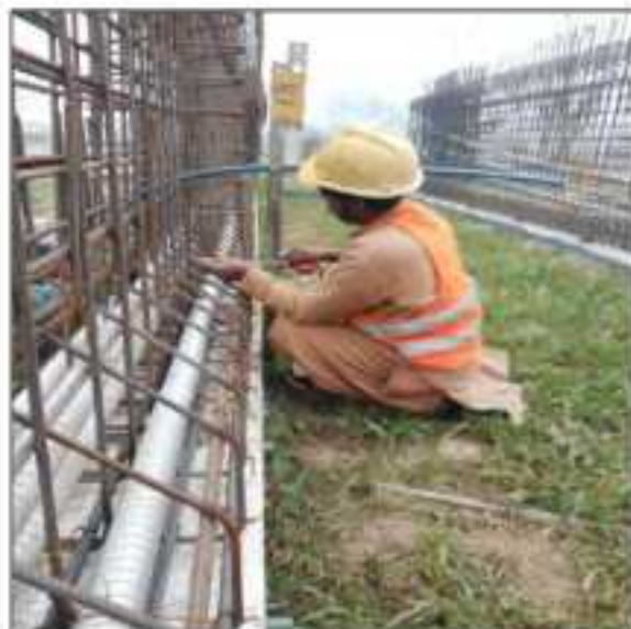
Picture 84: Steel reinforcement and profile of girder no 36 checking is in progress at flyover Sialkot.
