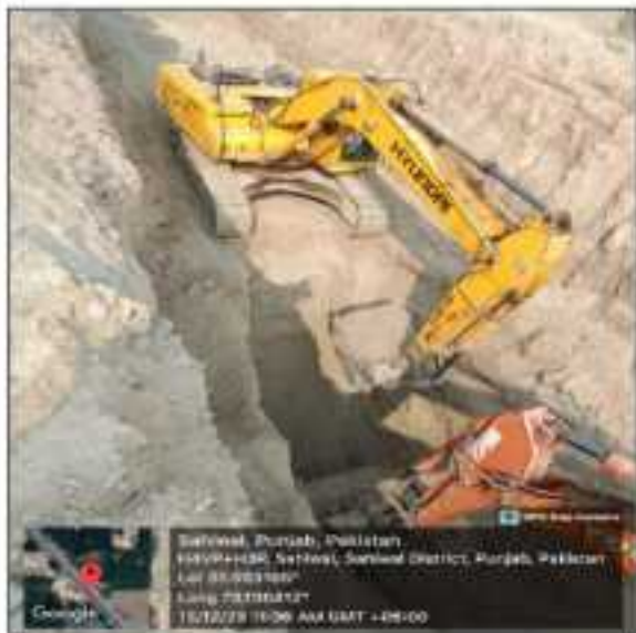
Picture 18: LOT-4 72 Inches Dia Sewer Pipes Laying at Pakpattan Road in progress Sahiwal
