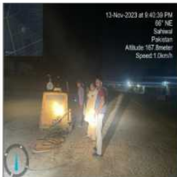
Picture 67: Laying of Asphalt Base course at Fateh Sher Road is in progress.
