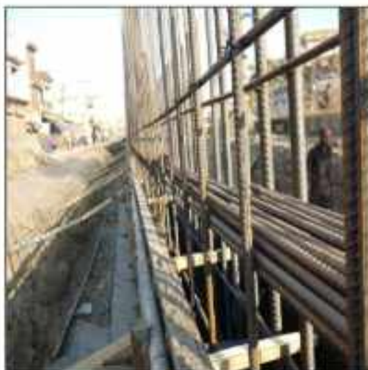
Picture 81: Form work of retaining wall is in progress at flyover sialkot.
