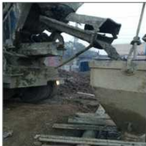
Picture 72: Pouring of concrete pile no 05 pier no 04 has been done at Flyover Sialkot.
