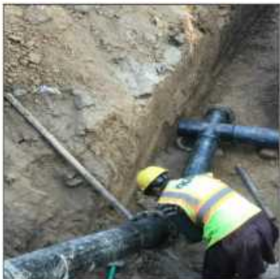
Picture 34: HDPE line laying in progress at T50 Islamia College LOT-4 Sialkot.
