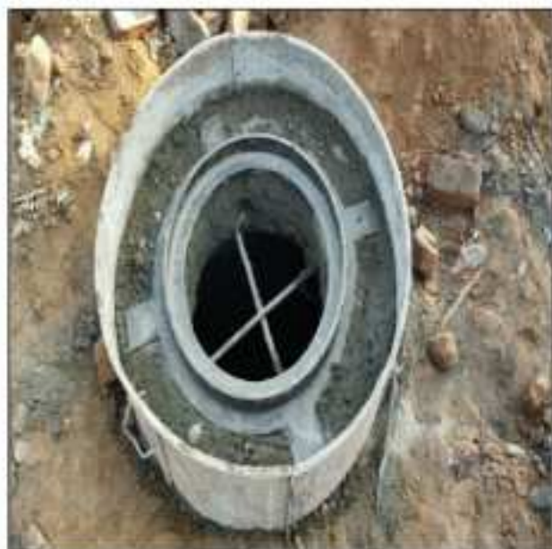
Picture 48: Neck preparation is in progress for MH#82 Khawaja Safdar Road 66 LOT-1 Sialkot.
