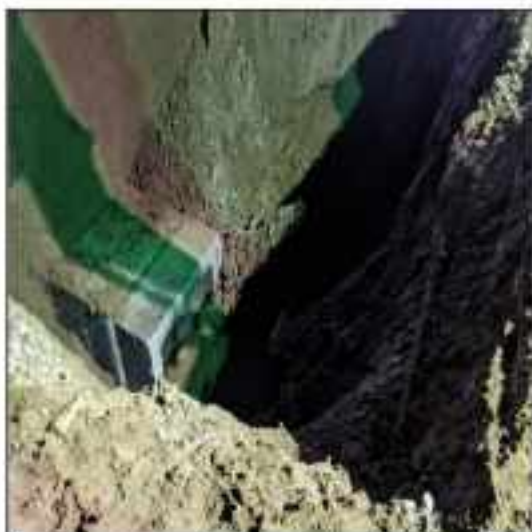
Picture 41: Excavation for MH#51 is in progress at single cell conduits line Murad Pur Chowk Marala Road LOT-2 Sialkot
