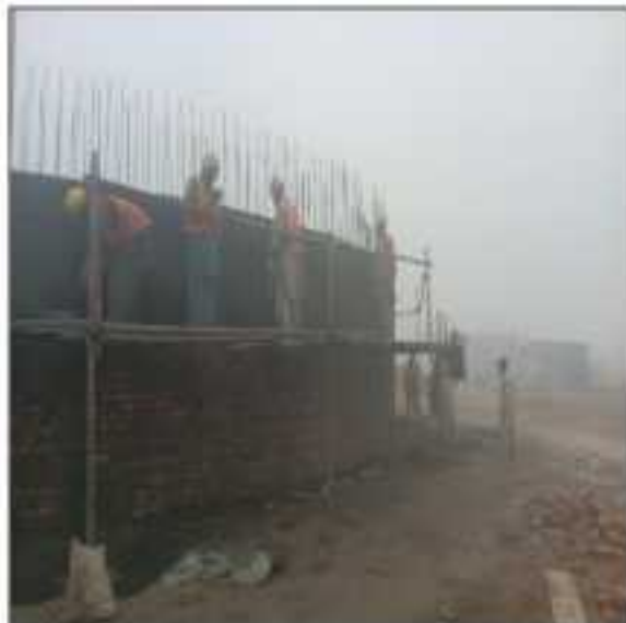
Picture 24: Plaster work of dry well is in progress of LOT-3 Disposal Station Sahiwal
