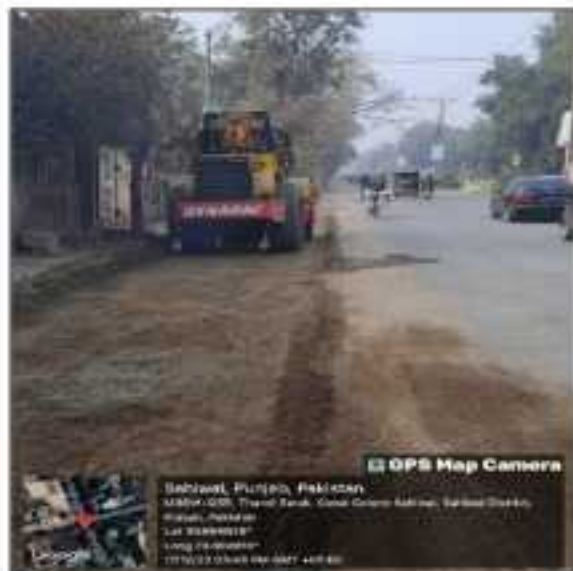
Picture 69: Arra Tulla Road Iqbal Road final Slip Road is in progress.
