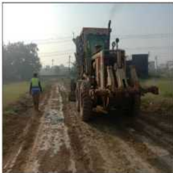
Picture 35: Clearing of ROW at Kacha portion is in progress at LOT-3 foreman Sialkot.
