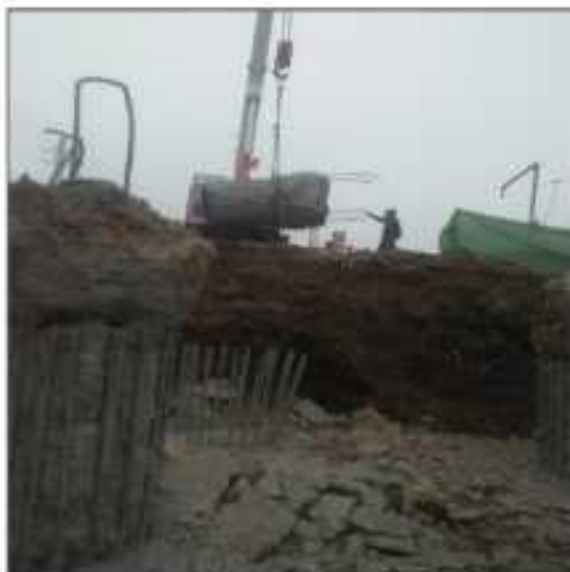
Picture 85: Dismantling of pile up to cut of level and removing of dismantling material of pile at flyover Sialkot.
