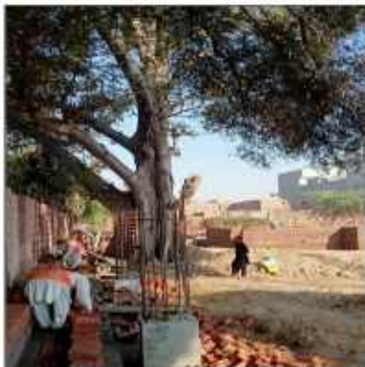
Picture 60: Boundary wall & column filling works at parking shed Fared Town Sahiwal.
