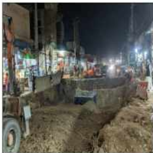
Picture 45: Back filling is in progress at MH#63 single cell conduits line Marala Road LOT 2 Sialkot.
