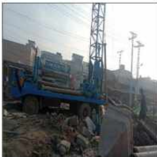
Picture 75: Drilling of pile is in progress pile no 08 pier no 04 at flyover Sialkot.
