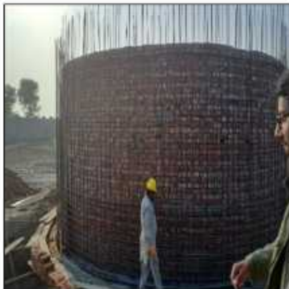
Picture 27: Brick work is in progress at LOT-3 Disposal Station wells of North Zone Sahiwal.
