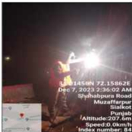
Picture 79: Steel cage fabrication and cage welding is in progress at flyover Sialkot.
