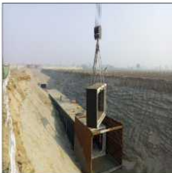
Picture 68: Conduit laying is in progress at Arra Tullah Road near Disposal Station LOT-3 Sahiwal.
