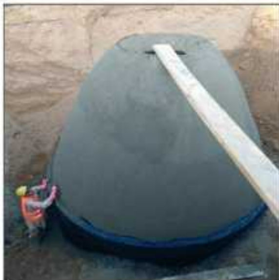
Picture 33: MH#90 outside plaster is in progress at Jail Road Chowk LOT-1 Sialkot.
